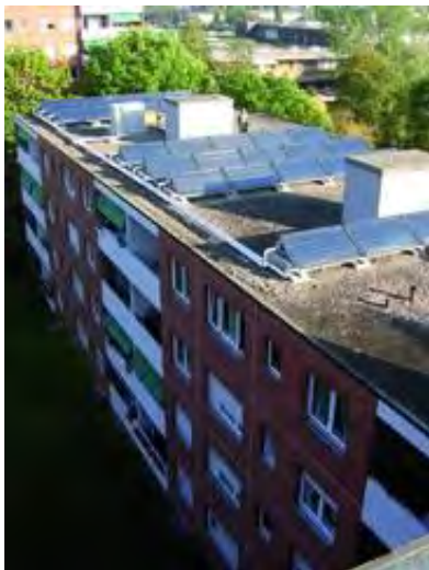
Figure 29. Picture of solar panels. Source:
